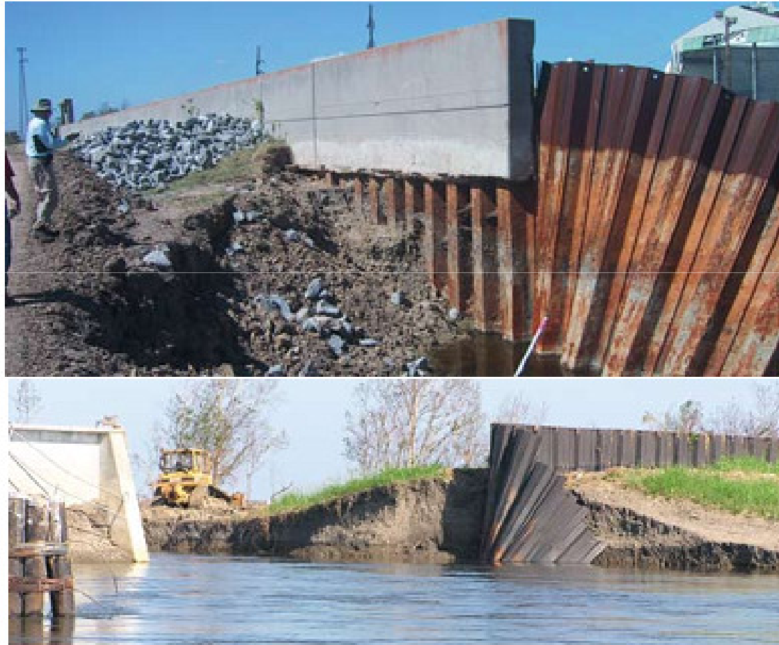
Failed I-Wall and Levee Sections
