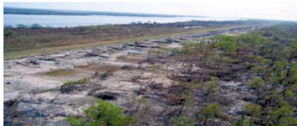
Obliterated Levee along the Mississippi River-Gulf Outlet
