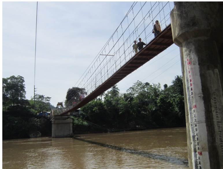
Fig. 11 - Hanging footbridge constructed after the destruction of the Bridge (Cabula-Maasin, Bukidnon province)
