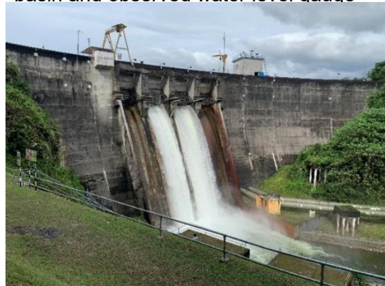
Figure 2-4 Klang Gate Dam and existing water level gauge (non-contact type)
