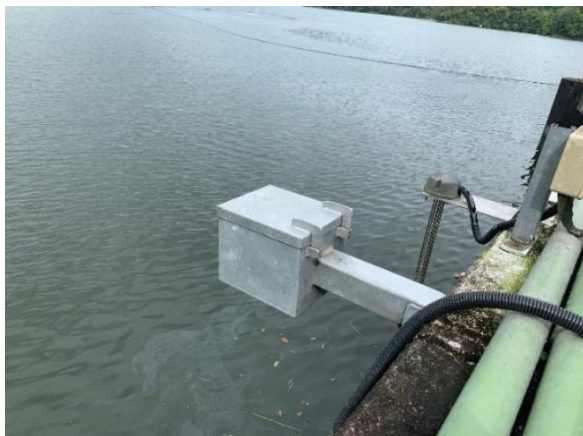
Figure 2-5 Klang Gate Dam and existing water level gauge (non-contact type)
