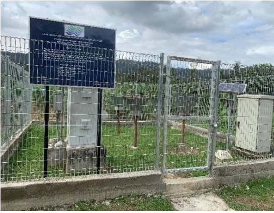
Figure 2-14 Sg. Langat Batu 12 Water Level and Rainfall Observatory and Water Level Gauge Sensor Section (Non-contact)
