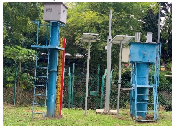
Figure 2-21 Water level gauge, siren, rain gauge and solar panel
