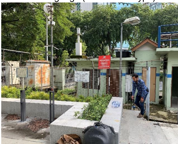
Figure 2-6 Sultan Sulaiman Bridge Water Level and Rainfall Observatory and Existing Water Level Gauge and Radio Velocity Gauge (non-contact type)
