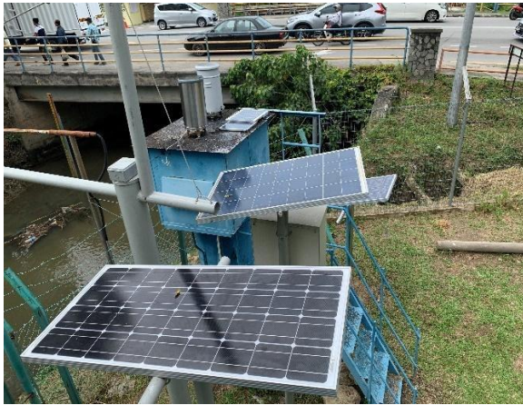
Figure 2-22(2) Water level gauge, siren, rain gauge and solar panel
