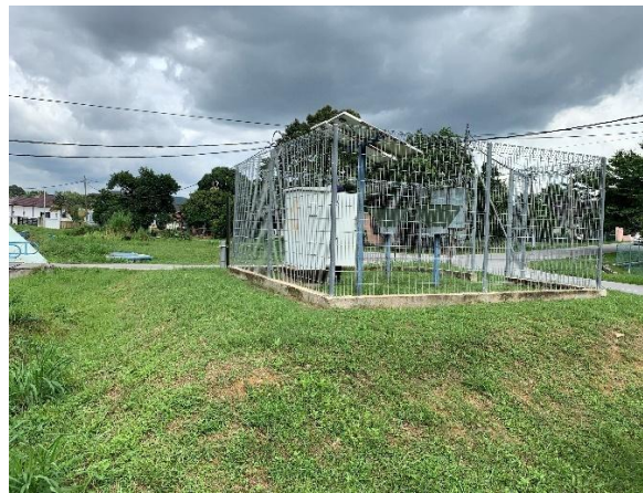
Figure 2-12 Kg. Sg. Kantan Water Level and Rainfall Observatory and Observation Section
