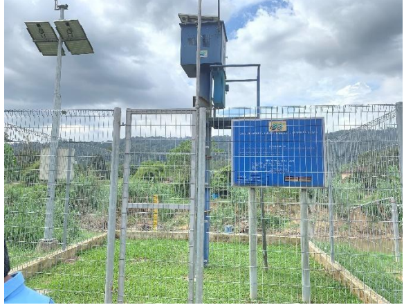
Figure 2-17 Web camera and siren device
