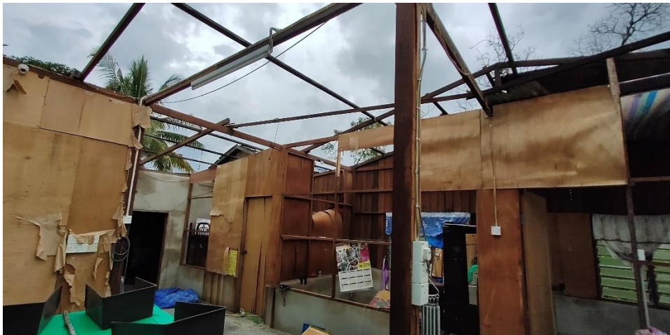
Storm causing damage to a house in Kedah
